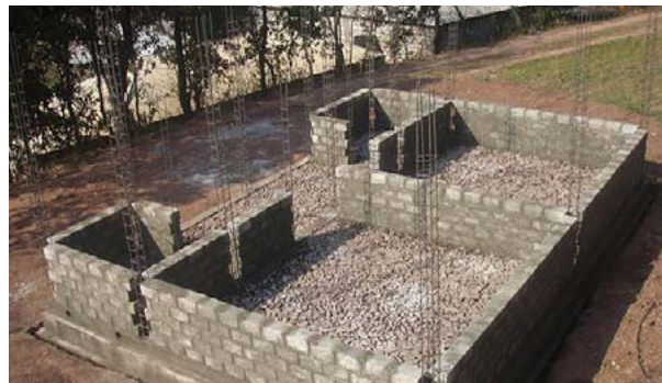
Model house constructed to generate training and information materials. Rising wall and steel reinforcement in confined masonry construction. Source: UN-Habitat.
