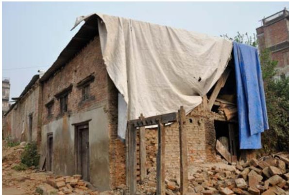
Tenants in earthquake damaged historic buildings, unable to carry out repairs and ineligible for financial assistance. Source: World Bank.
