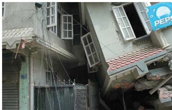
Individual building collapse in Kathmandu after the 2015 earthquake and damaged caused to the neighbouring building. Property insurance in urban areas needs to take account of settlement as well as building and risk factors. Source: Shelter Cluster Nepal.
