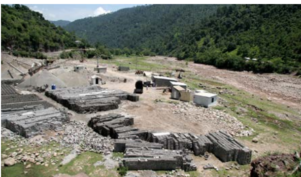
Expansion of concrete block production capacity to meet increased demand in reconstruction. Source: UN-Habitat.
