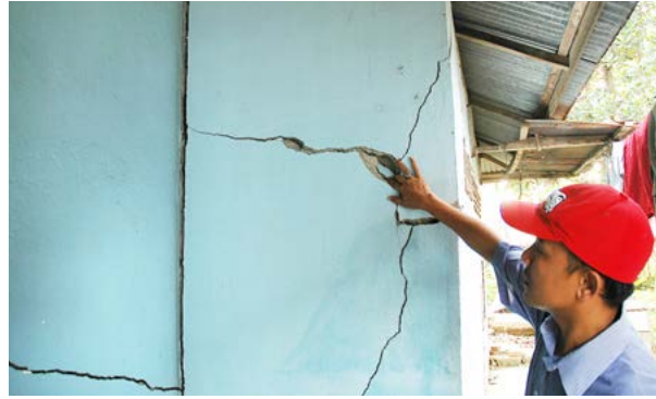
Assessing cracks in building for repair or reconstruction. Indonesia. Source: UN-Habitat.
