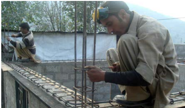
Technical assistance mobile steel fixer demonstrates steel band corner details at lintel level for household and masons to replicate. Source: UN-Habitat.
