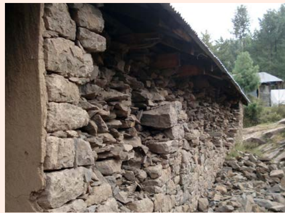
Earthquake damaged wall showing typical pattern of delamination. Pakistan. Source: GOAL Ireland.
