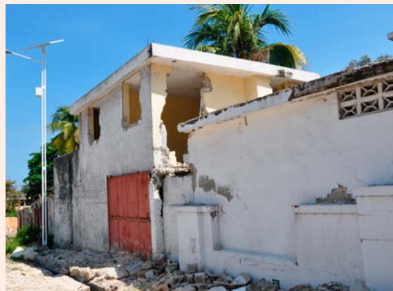
Housing damage after the 2010 earthquake Port au Prince Haiti. Source: UN-Habitat.
