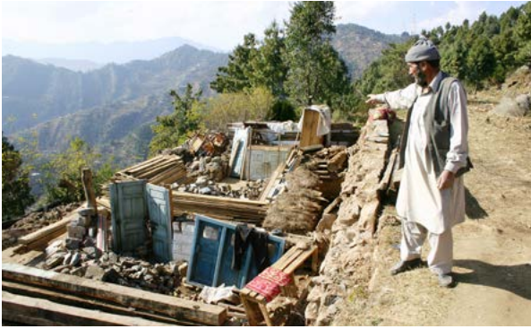
Household saves all roof timbers, windows, and doors in preparation for rebuilding. Source: Robbie Ryan/GOAL.
