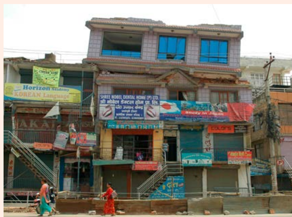
Individual building failure. Top story pancaked onto the three lower stories. Source: Shelter Cluster.
