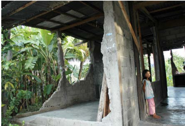
Children playing in unsafe damaged buildings, out of school after disaster and uncertain of their homes and futures. Indonesia. Source: UN-Habitat.
