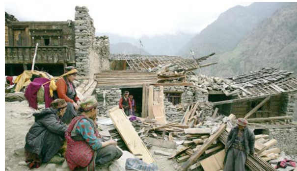
Households in a remote village in Nepal used shelter cash assistance to purchase permanent building materials and to start work on repairs to damaged buildings a few weeks after the 2015 earthquake. Source: GOAL.
