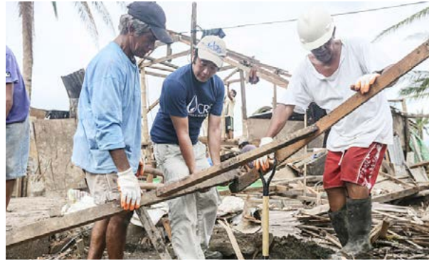
Dismantling damaged houses and salvaging materials after cyclone Haiyan (Yolanda). Source: CRS.
