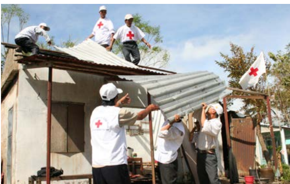
Red Cross team helps with repairs to roof to make the house habitable after cyclone damage, Vanuatu. Source: IFRC.
