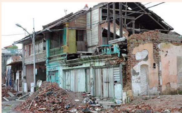
Historic shop houses damaged by 2009 earthquake in the centre of Padang, Indonesia. Mainly absentee property owners. Source: UN-Habitat.
