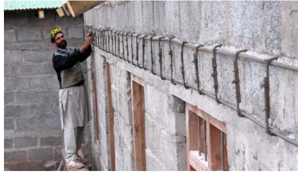
Retrofitting an external band to make substandard new construction safer. Technical assistance to diagnose and address emerging problems. Source: UN-Habitat.
